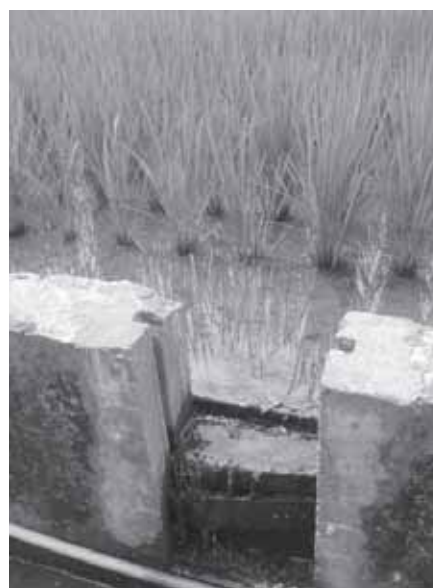
Fig.12 Paddy water drainage
