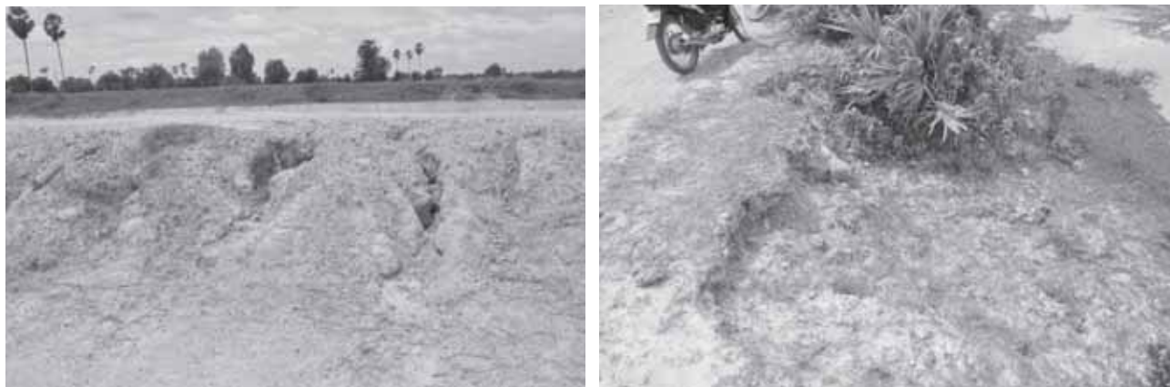
Figure 1: Canal bank erosion at model sites
