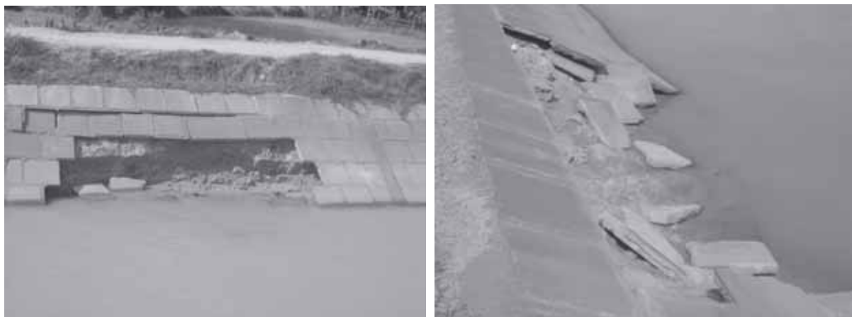
Figure 3: Canal structure failure at irrigation model site
